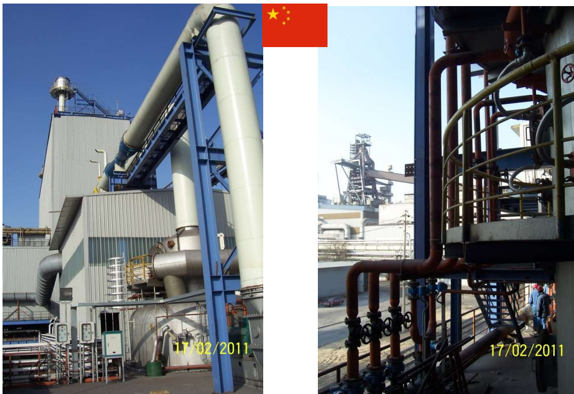
Shaft Furnace GCP (processing residues from stainless steel production) in Taiyuan (China)
