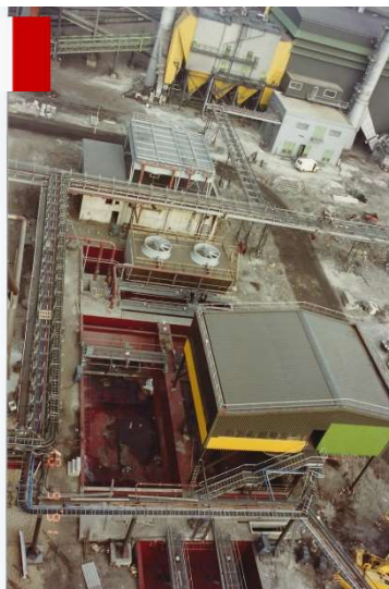
GCP of a fully enclosed AC-SAF (FeMn/SiMn Furnace) in Dunkerque (France)
