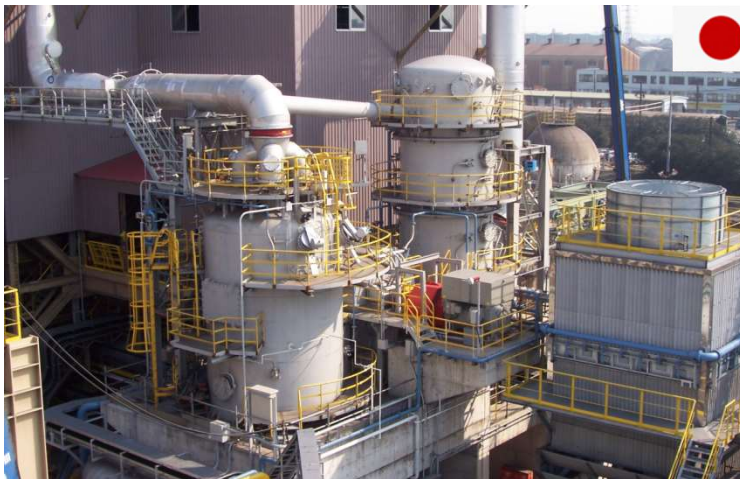
Shaft Furnace GCP (processing residues from steel production) in Nagoya (Japan)
