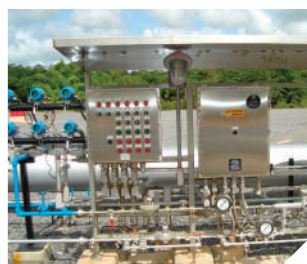
Painel de controle Control panel
